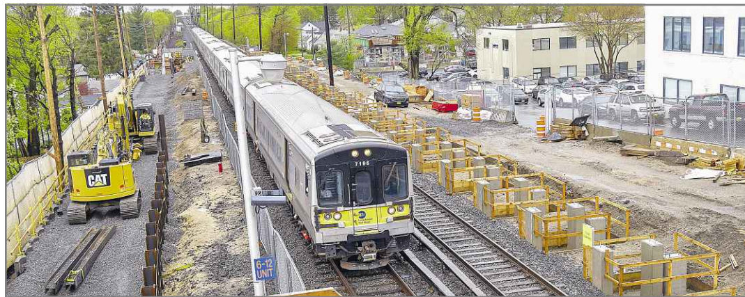
The capital budget includes funding for the Third Track project between Floral Park and Hicksville.
