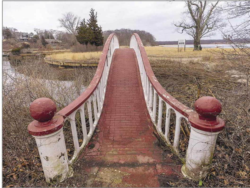
The rebar-concrete Ransome Japanese Bridge was named to the National Register of Historic Places.
